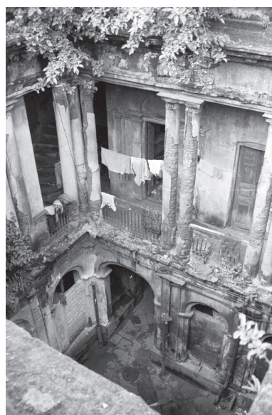
Fig. 16: Parapet detail of dilapidated Dolls House.
